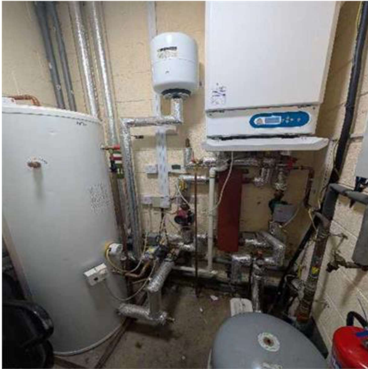
Key Stage 1 plant room
